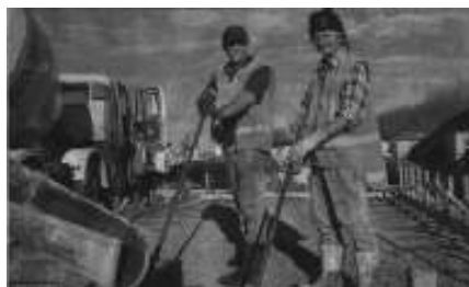
Ashburton resource recovery park workers Jonny Bowman (left) and Gerry Tinning are all set to help with the pouring of the glass-containing test slab.
