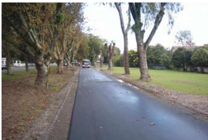
Palmerston North City Council worked with Higgins Aggregates to make this cycle track which uses recycled glass as an aggregate material.
